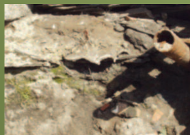
BURIED ASBESTOS SHEETS
