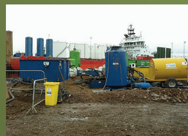
ALL 3 TREATMENT KITS & GENERATOR
