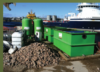
SOILUTIONS TREATMENT EQUIPMENT
