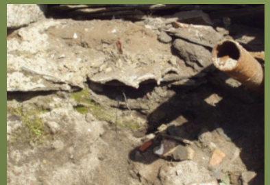
BURIED ASBESTOS SHEETS
