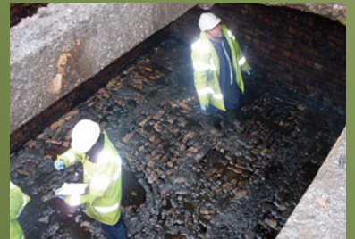
TANKS FOLLOWING OIL & TAR REMOVAL
