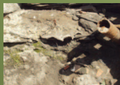
BURIED ASBESTOS SHEETS
