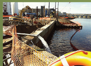
DE-WATERING DISCHARGE WATERS
