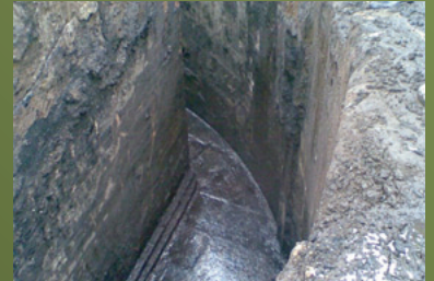
GAP BETWEEN TANK AND GAS HOLDER
