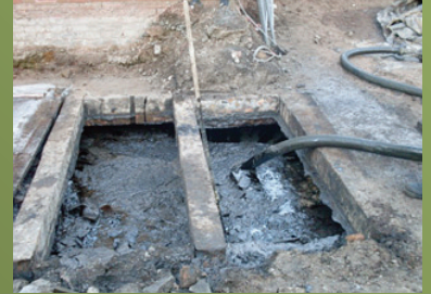
EXPOSED TANKS FILLED WITH OIL & TAR
