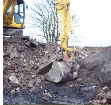
A recent excavation & removal job of ours, treatment was not a practical option.
